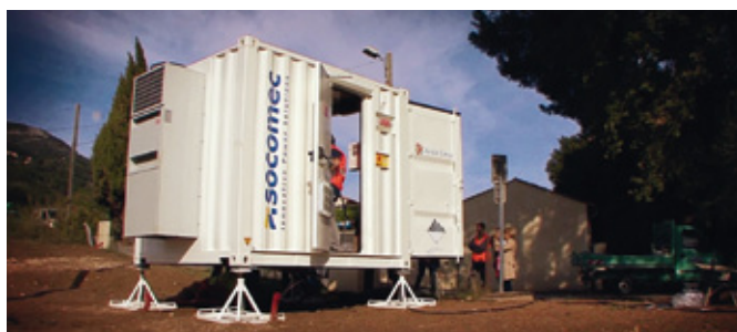
Easy to use, this 33-kW storage container is installed on the low-voltage network.
